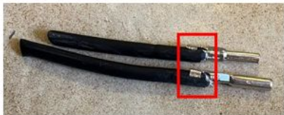
Incorrect terminal crimping:
